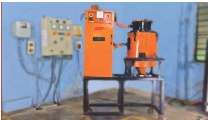
Bry-Air Dryer working since 1995
