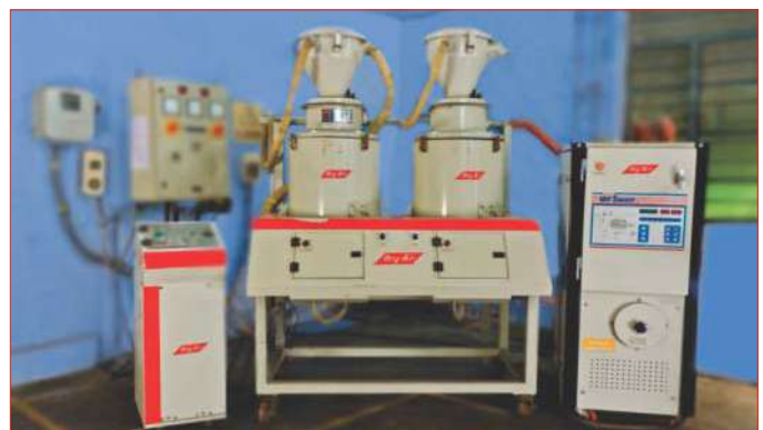
Bry-Air Honeycomb Resin Dryer recently installed
