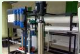
Waste Water & Sewage Treatment Plant
