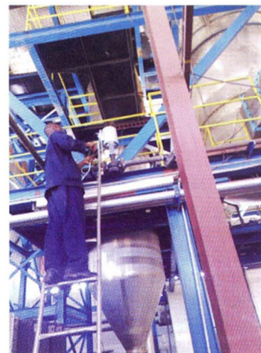
Figure 4: View of fluidized bed dryer
